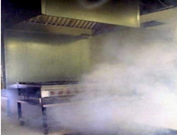
Photo 5 Smoke From Backdrop Plenum
