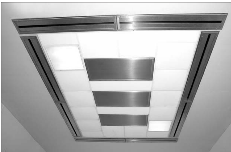
Photo shows standard 12 x 8 Steri-System module installed in the Nailor Air Distribution laboratory.
